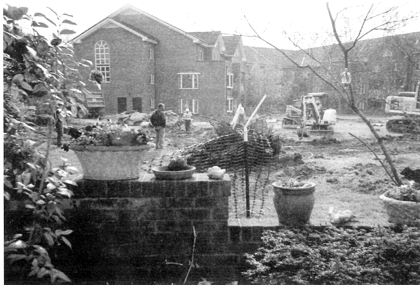
Southminster under siege by construction. Residents look forward to the completion of the new facilities.
